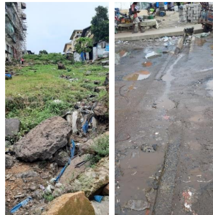
Photo 2: Open Space between Water Street and Front Street (left), Photo 3: Clogged drain at Water Street towards Mesurado Estuary (right)
