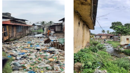
Photo 2: Garbage blocking drainage through culvert underneath UN Drive (left), Photo 3: Outlet Duala Market towards St Paul River (right)
